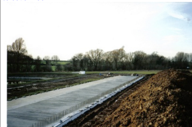
Completed sub-slab – Note soil on left to be used later to cover roof
