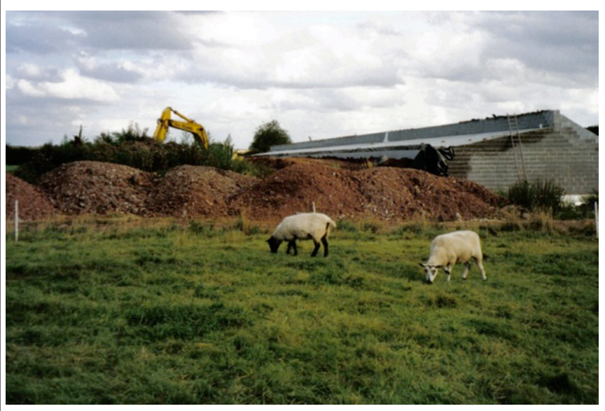
Soil being placed on roof and returning green footprint, to be used in future years for sheep grazing
