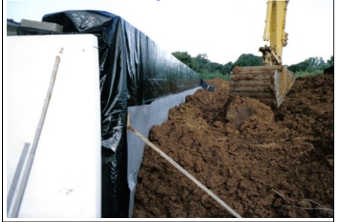
Back wall infill – Note the Geofin layer (paler coloured sheet between earth and dpm)
