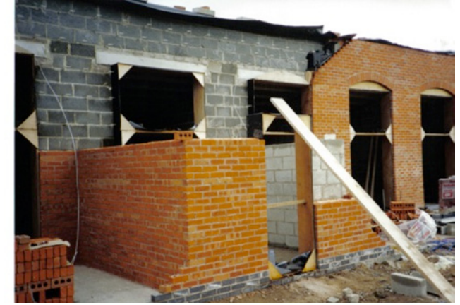
Front wall and porch construction – note plastic wall ties from inner leaf of blocks
