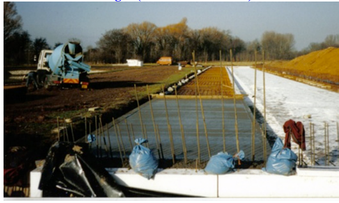
Main slab partially complete. Note steel mats in distance and insulation on right (main house section)
