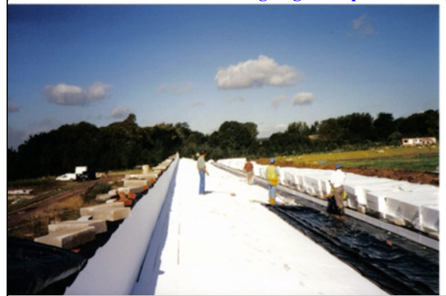
Dpm being laid on thin insulation off cuts – Main insulation blocks on side waiting to go on dpm
